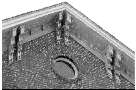
Detail of the Hilt-Keator House roofline, with elaborate brackets and oculus window
