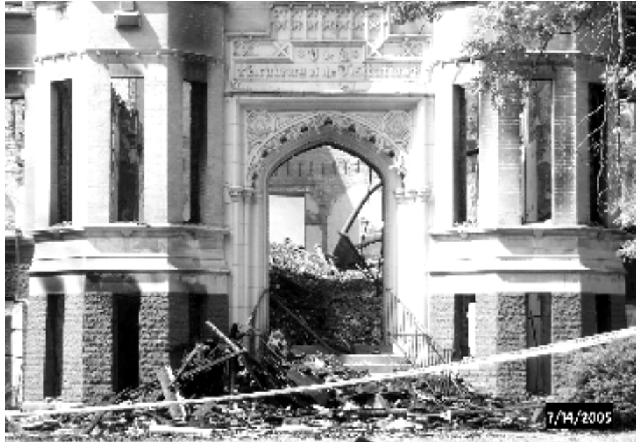
The Entrance Arch still stood after the devastating fire which destroyed much of the historic Villa de Chantal in July 2005
